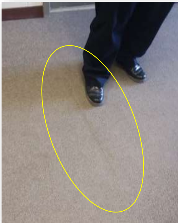
↑ Heaving in concrete floor of police station entry, identified spring 2018.
