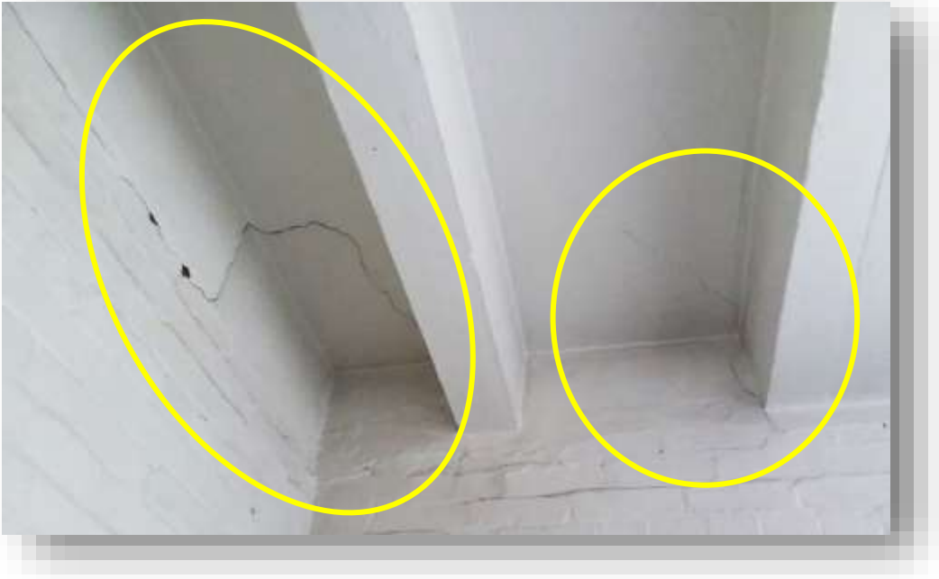
Interior cracking in concrete ceiling and masonry wall near southwest corner of police station. →
