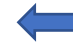
Loss of thin bricks from exterior of police station. Occurred prior to September 2015 2
