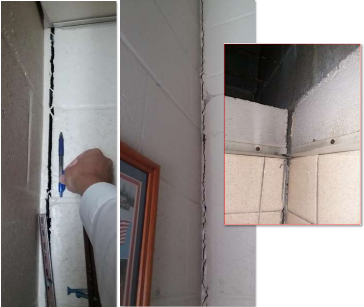
Pictures taken August 6, 2019 of structural fissures at the fire station. Pictures taken within the common room, sleeping quarters and bathroom located along the south and west exterior walls.
