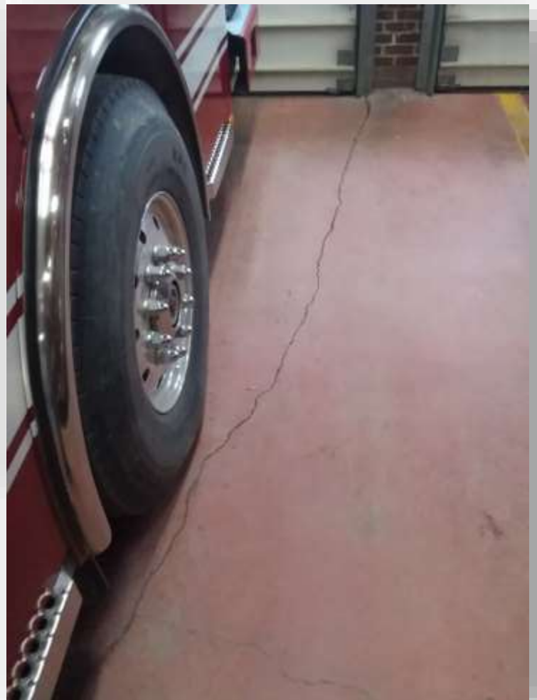
Increased floor settlement and cracking in fire bays due to heavier weight of apparatus. →
